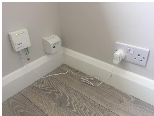
Figure 3 – ONT, Power Supply and Internal Wiring
