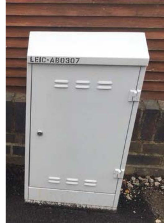
Street side cabinet
